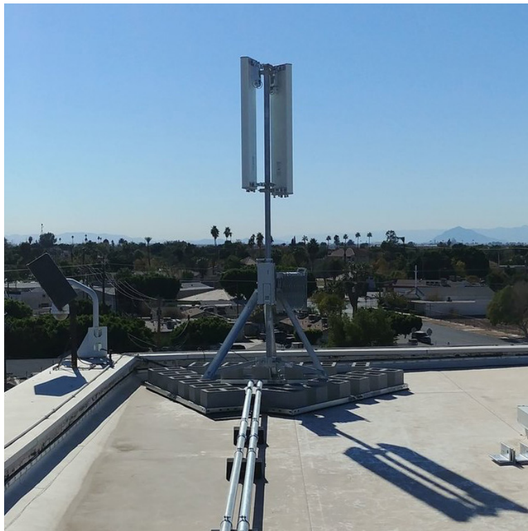
A “school-as-tower” installation at Brawley High School.
