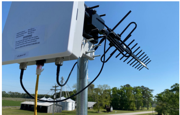
TVWS CPE installed near Engelhard, NC.
